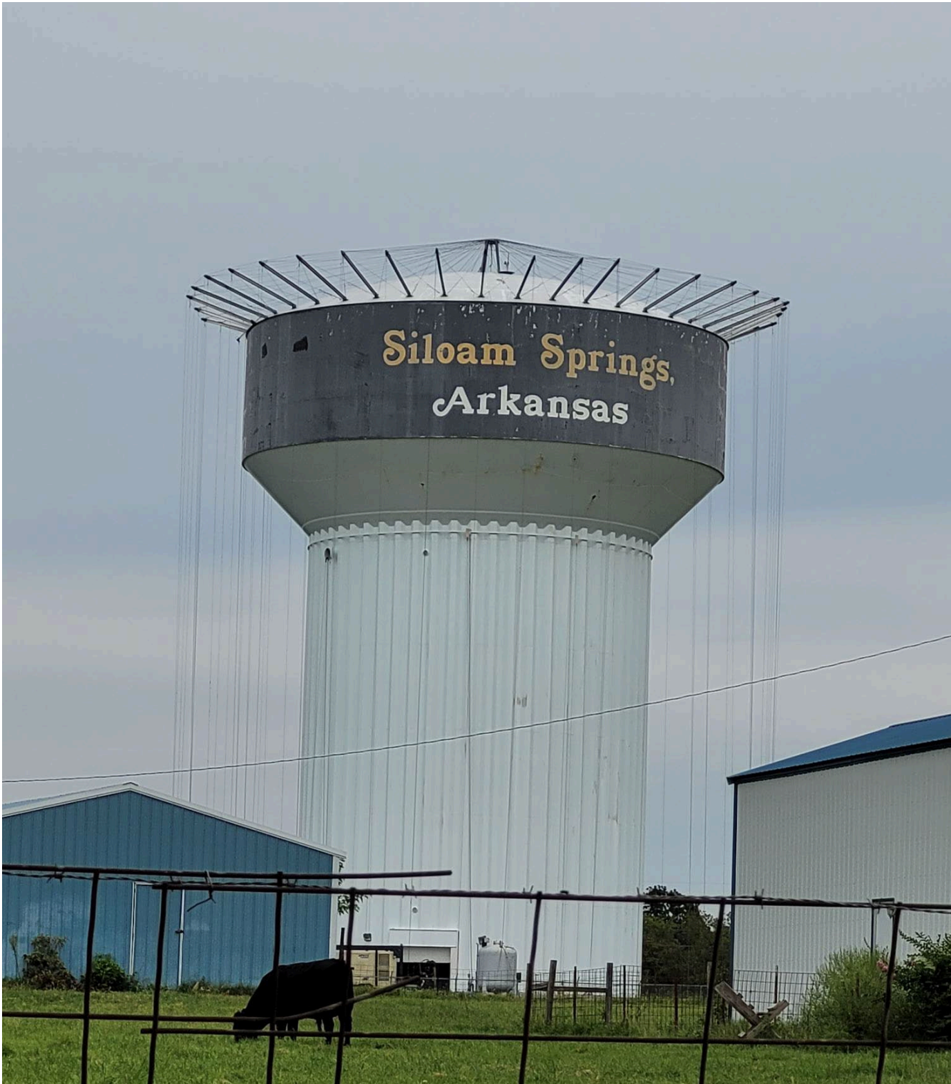
Rigging for curtain
